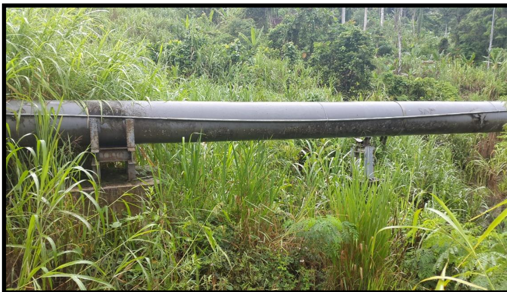
Photo 5-2 Ramu NiCo slurry pipeline
