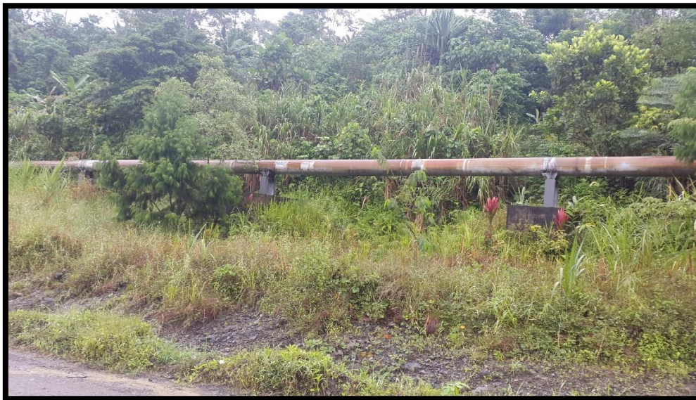
Photo 5-1 Ramu NiCo slurry pipeline
